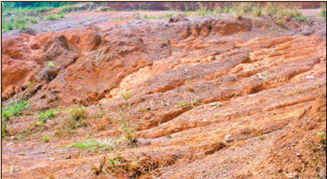
Soil Erosion along Sir Apollo Kagwa Road in Kampala. (cover photo) Source: New Vision Library
