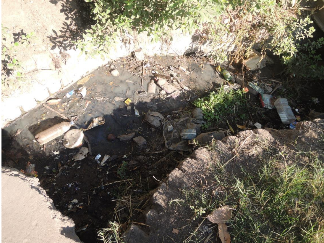
Figure 9: hydric facilities in one of the miners' villages
