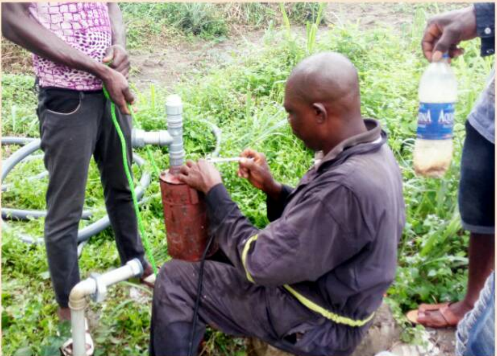
Installation of Borehole Pump at Okwabude PHC Facility during MNCH Project Implementation
