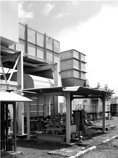
Lahmeyer provides advisory services for the conversion of a power plant in Maputo in Mozambique
