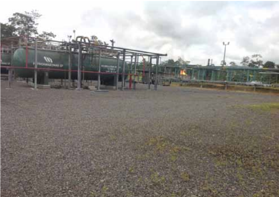
Figure 4: Gas Flaring at the Central Processing Facility (CPF), of Petroamazonas' Block 15, Amazon Region, Ecuador, Nov. 2016
