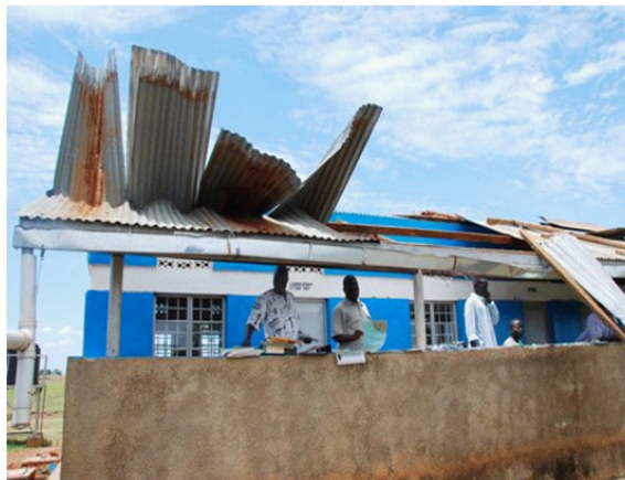
Figure 4: Atiak Health Centre operating under dangerous conditions. The health centre was destroyed after a heavy storm.
