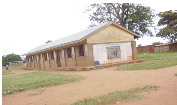
Figure 3: School structures that are slowly running down without repairs at Koch Goma Central Primary School.
