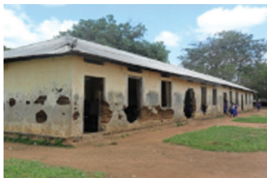
Figure 4: Dilapidated Structure at Angopet Primary School in Gweri Subcounty
