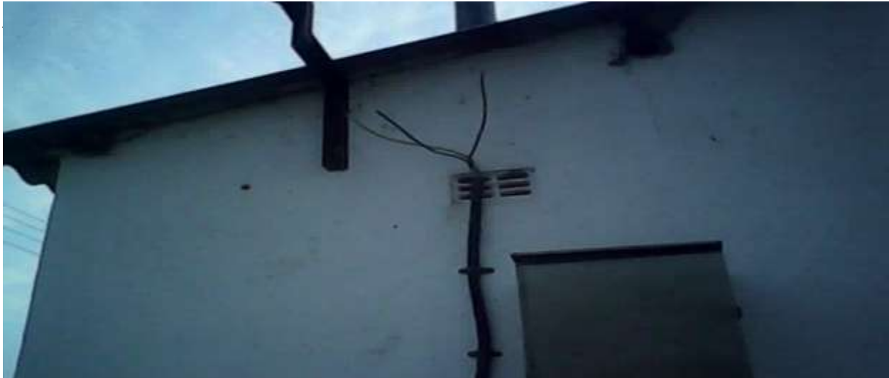
Abandoned electrification project that was started by Bayrich Enterprises in 2011 for Madzivire Primary school
