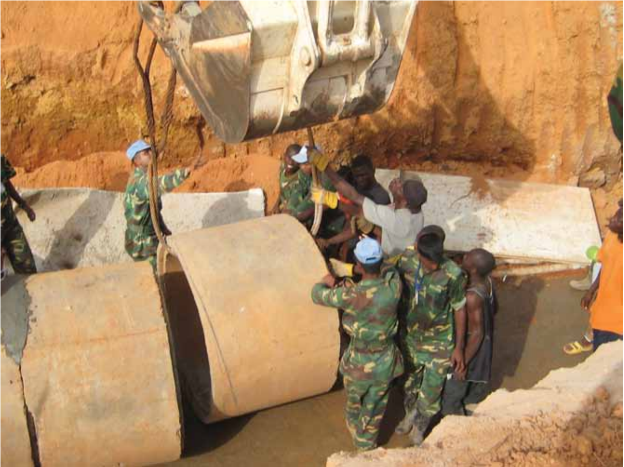
Liberian Ministry of Public Works personnel receive on-the-job training in culvert restoration from Bangladeshi engineers.
